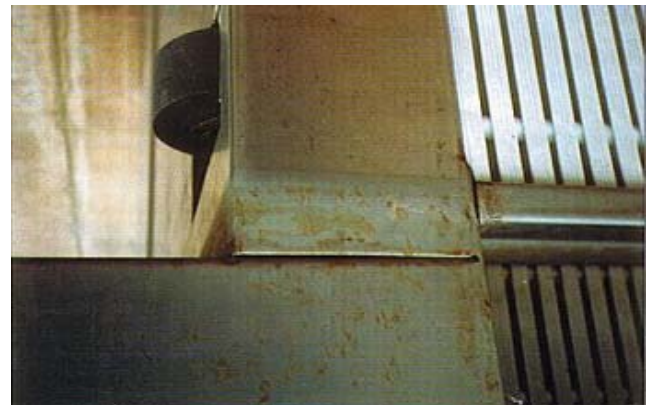
Top: Ease of movement of 25m long bulkhead. Above: Example of corrosion on stainless steel bulkhead.
