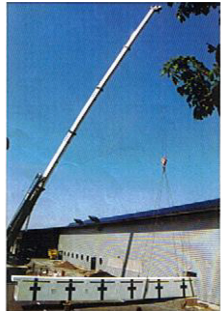
Above: 25m long bulkhead, 1.5m wide being lifted into Tollcross Park Leisure Centre, Glasgow
